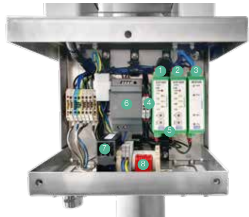
Slave unit at the motor drive side
