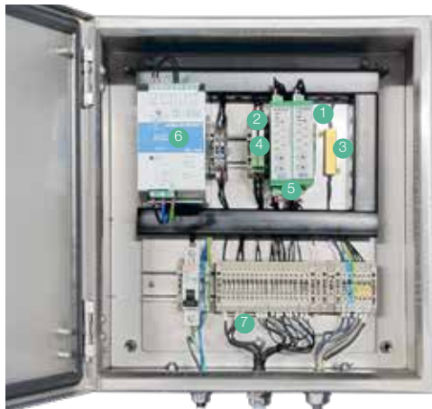
Master unit at the SCADA side
