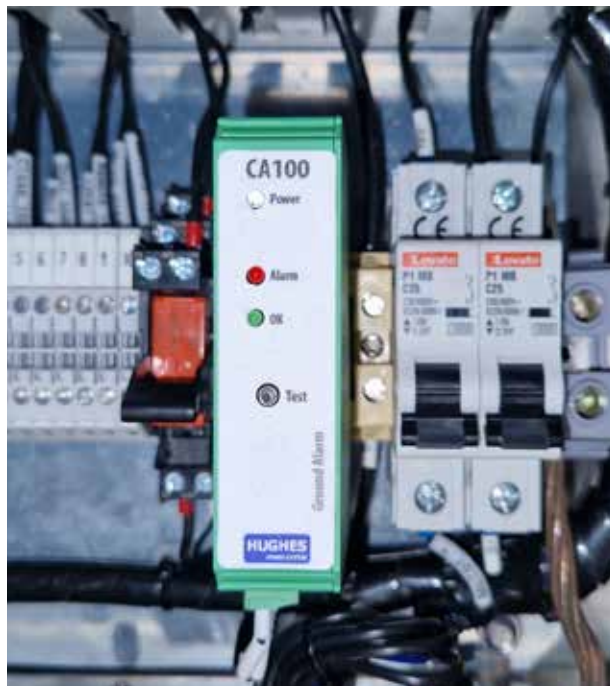
Installation in the motor drive cabinet
